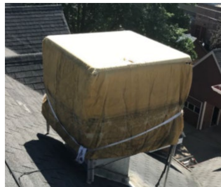
Example Evaporative Cooler with Cover
